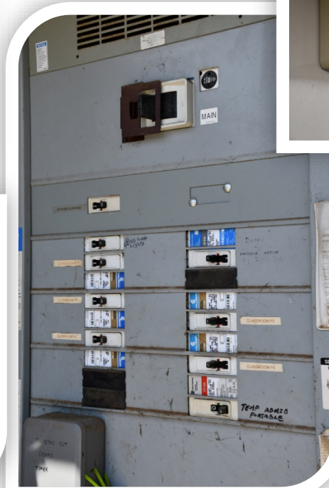
Outdated electrical systems
